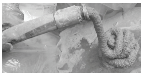
Fig.3 Pumping of Höganäs Pump LC50
