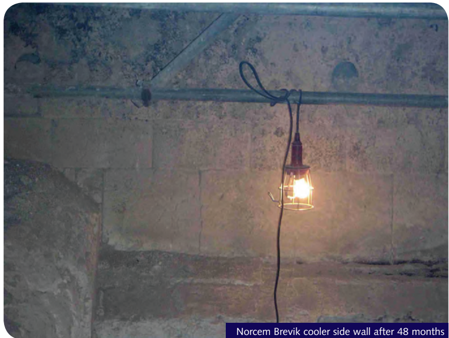
Norcem Brevik cooler side wall after 48 months
